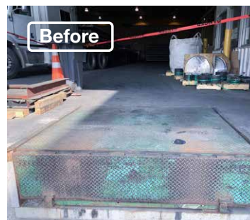
Damaged concrete and missing bumper
